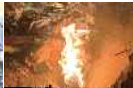
Fire on a conveyor belt in an incineration plant
